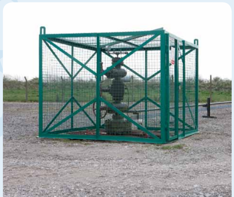
The well head at our Elswick site .
